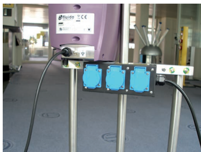
Power strip for hospital equipment
